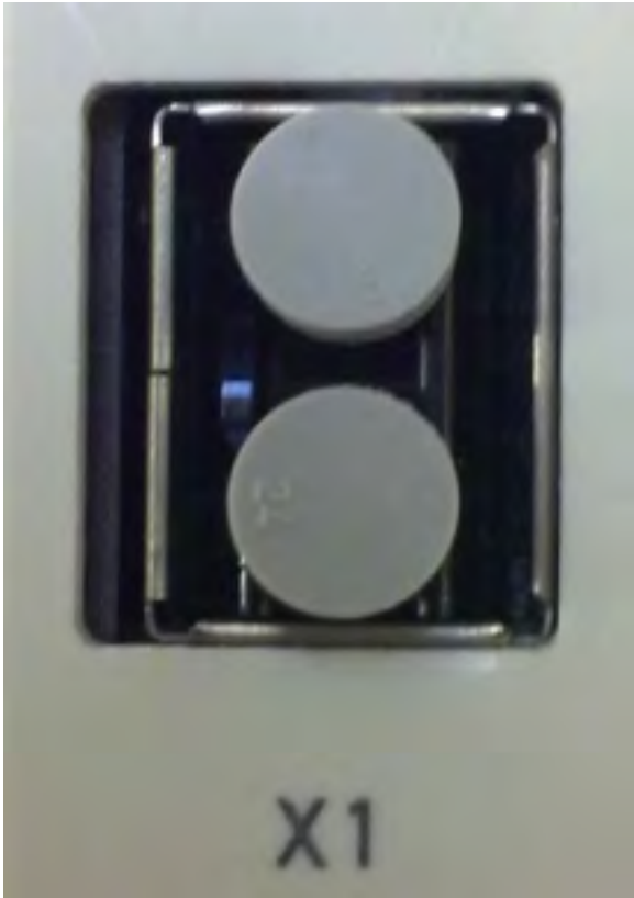
Figure: Blind plugs in unused sockets
